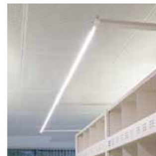
LED Lighting Luminaria Luminaire
